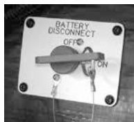
Battery Disconnect Switches
