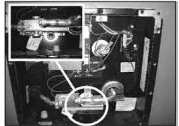
Fig 1: Water heater drain plug
